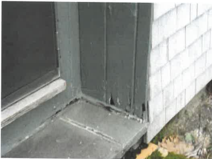
Trim rot noted
