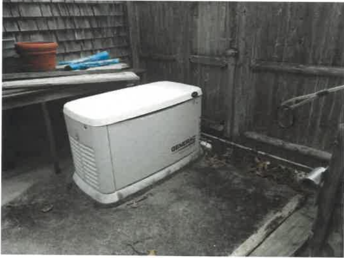
Whole house generator
