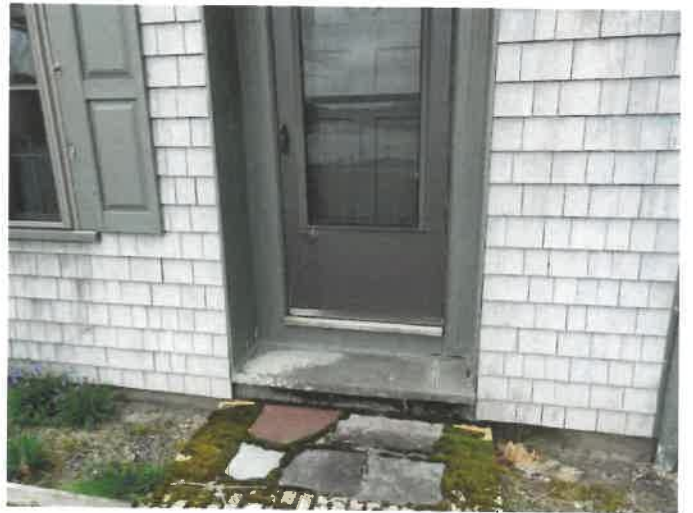
Trim rot noted
