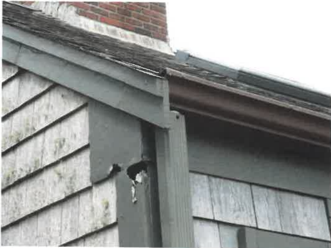
Trim rot noted
