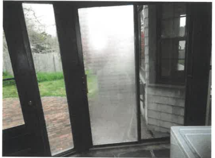
Slider glass needs replacement
