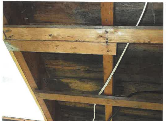
Possible Mold noted in unfinished attic
