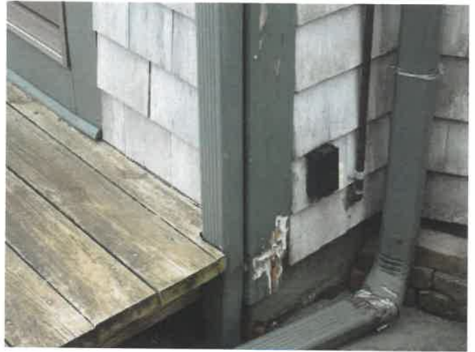
Trim rot noted
