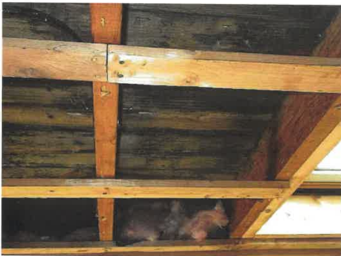
Possible Mold noted in unfinished attic
